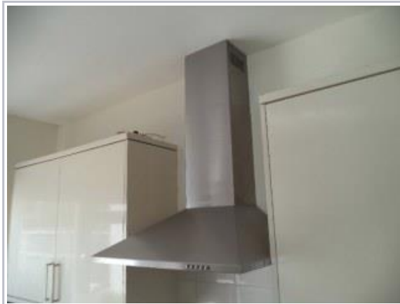
Inward venting extractor
