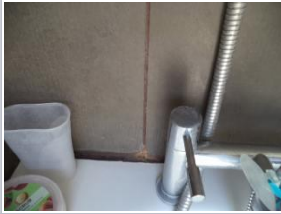
Deteriorating bath seal
