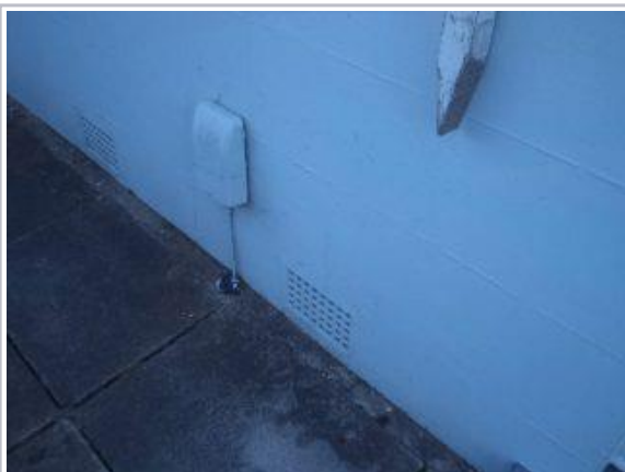
Airbricks at front good but limited at the rear
