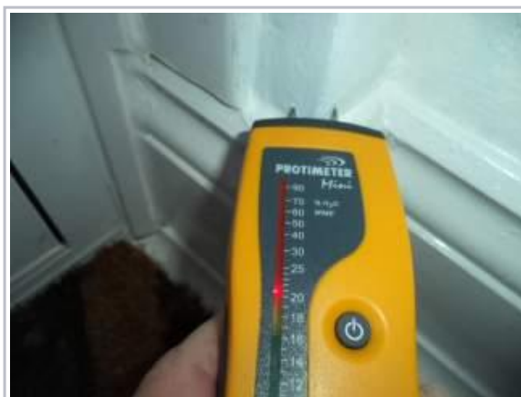
Damp in hall
