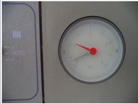
Low boiler pressure
