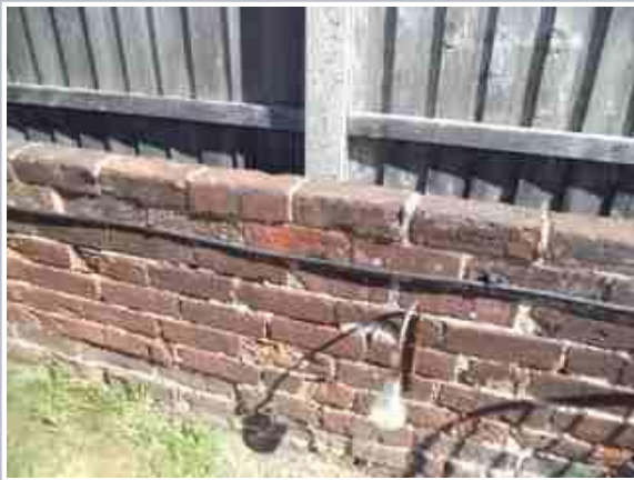
Poor boundary walls
