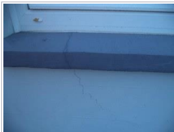
Cracked cill and render
