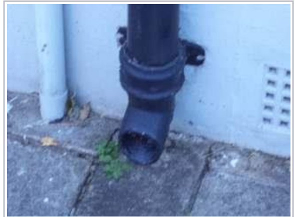
Gutter discharges onto the pavement
