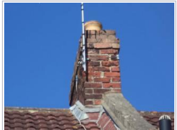
Poor pointing rear of chimney
