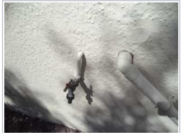
Uninsulated outside tap
