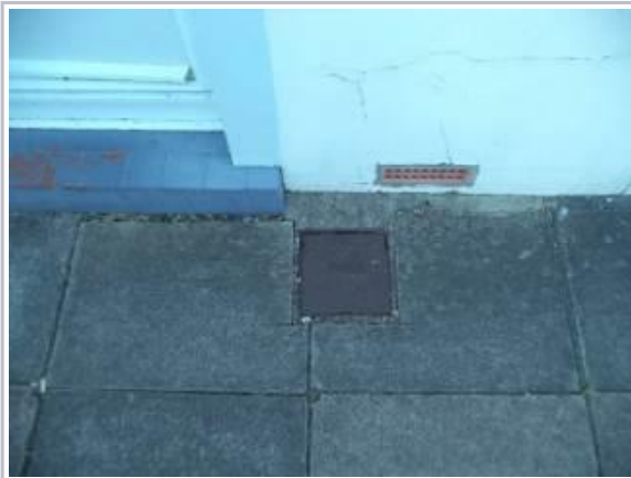
Pavement stop cock
