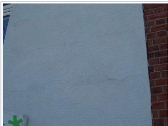
Wall tie related cracks
